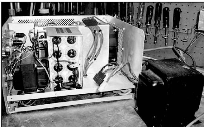
Figure 1 — The connectorized transformer, new capacitor bank and diodes.
