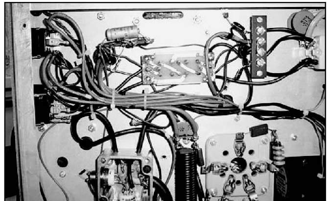
Figure 2 — Underside view of SoftStart and primary wiring.
