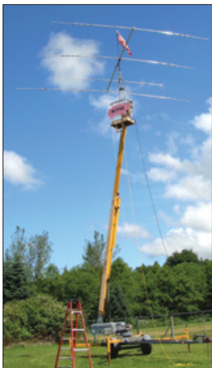
The flag is flying, and so are the pigs, atop one of the makeshift towers at the site of the Stanwood Camano ARC, W7PIG, near Stanwood, WA.
